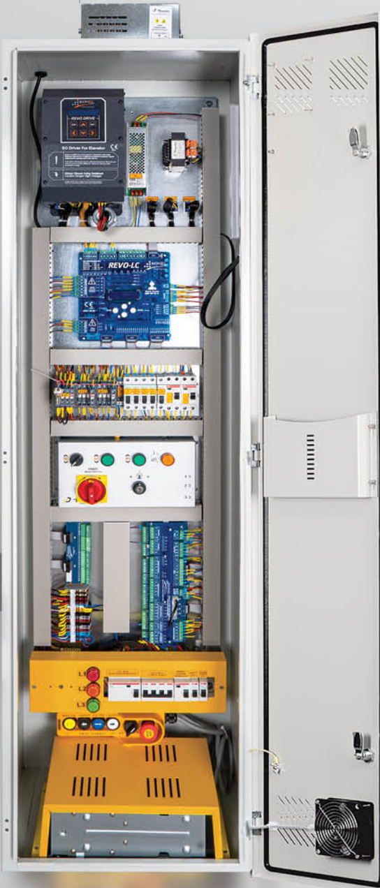
Dişlisiz Pano Gearless Control Panel
